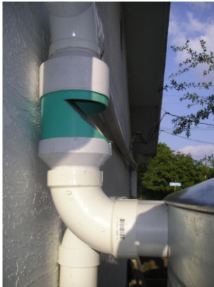
Figure 16. Primary filter installed at tank inlet
