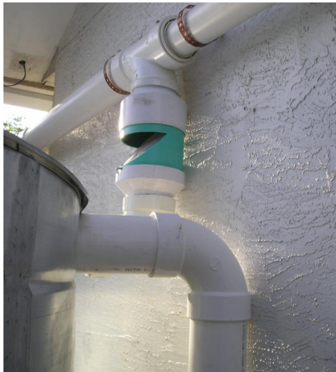
Figure 19. Overflow pipe, next to primary filter, in final system.
