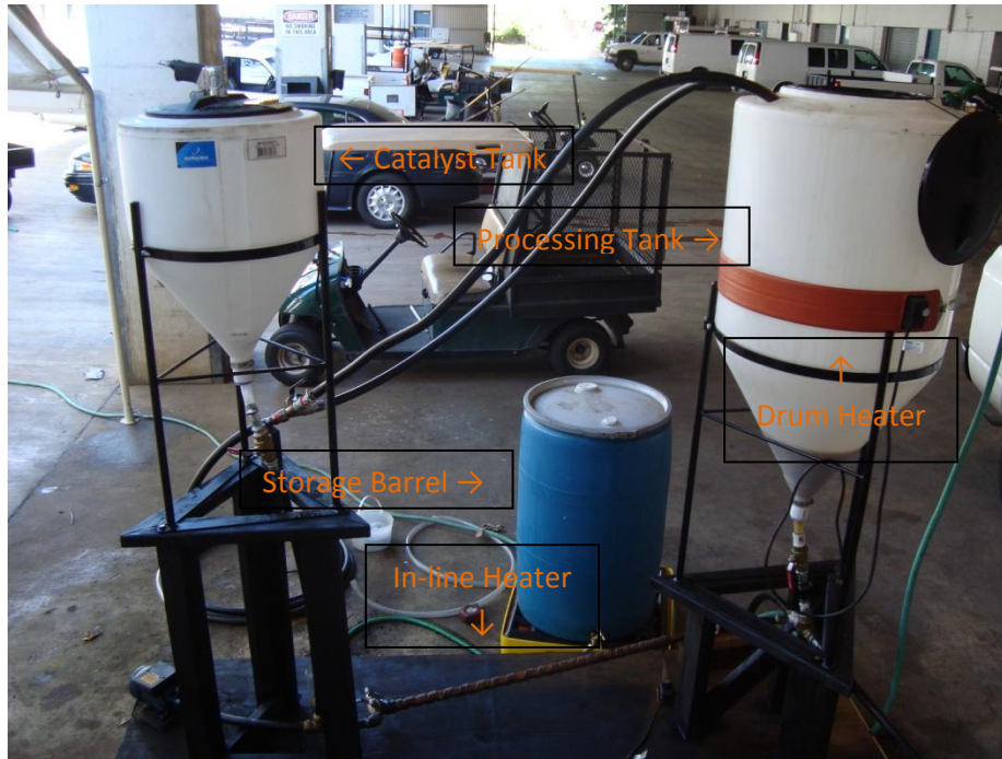
Figure 1 TUBI Biodiesel Processing System
