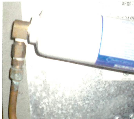
Figure 2: The outlet of the filter.
