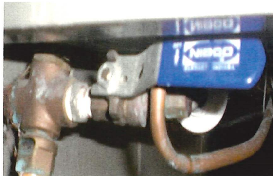
Figure 1: Retrofitted piping leading to the inlet of the filter.
