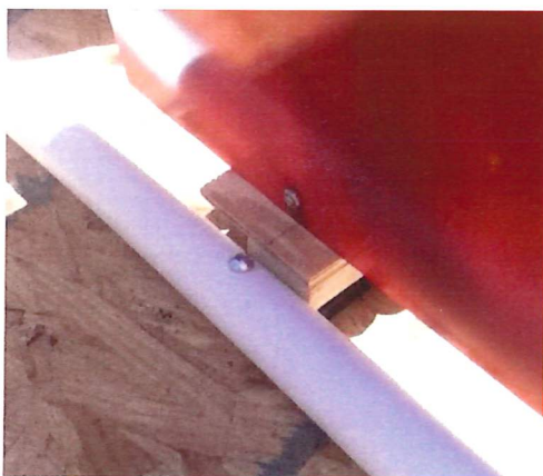
Figure 12: Target flush with PVC track
